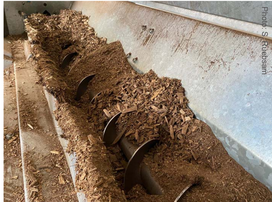
Discharge screw conveyor of the bioenergy plant in Altlandsberg with small particles/dust from low-quality wood chips
